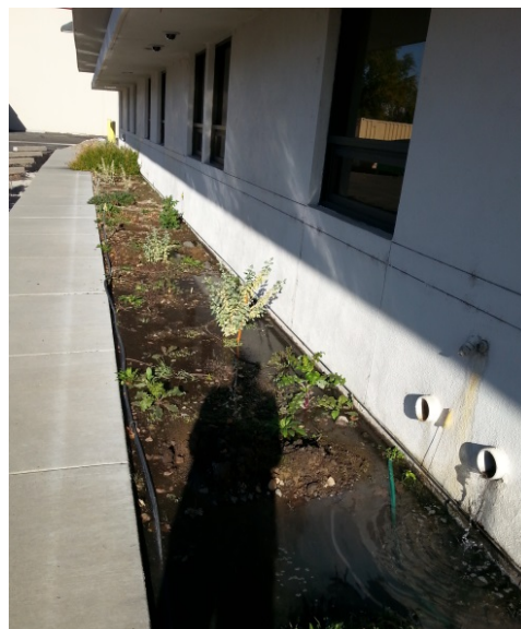
Figure 1. Flooding of the demonstration garden bed due to a break in the wall faucet in late summer 2015. Flooding was most acute within a meter on either side of the wall faucet. Soil moisture levels were elevated in a decreasing gradient with increasing distance from the irrigation water source.
